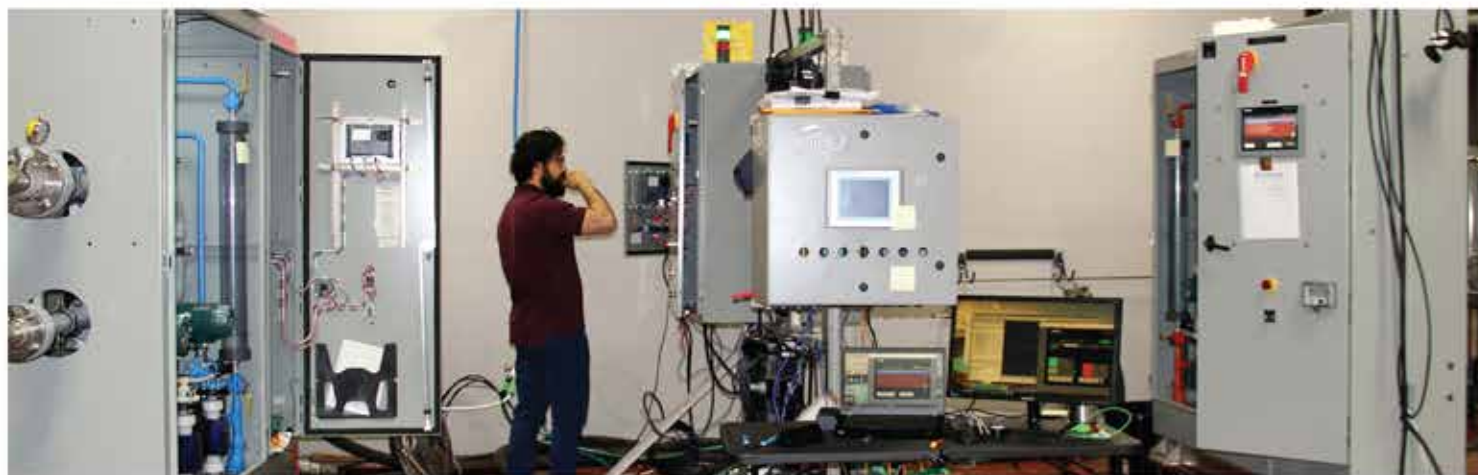
Electrical engineer performs FAT on the Ecochlor treatment system generators at the new ProFlow manufacturing factory in North Haven, Connecticut USA.
